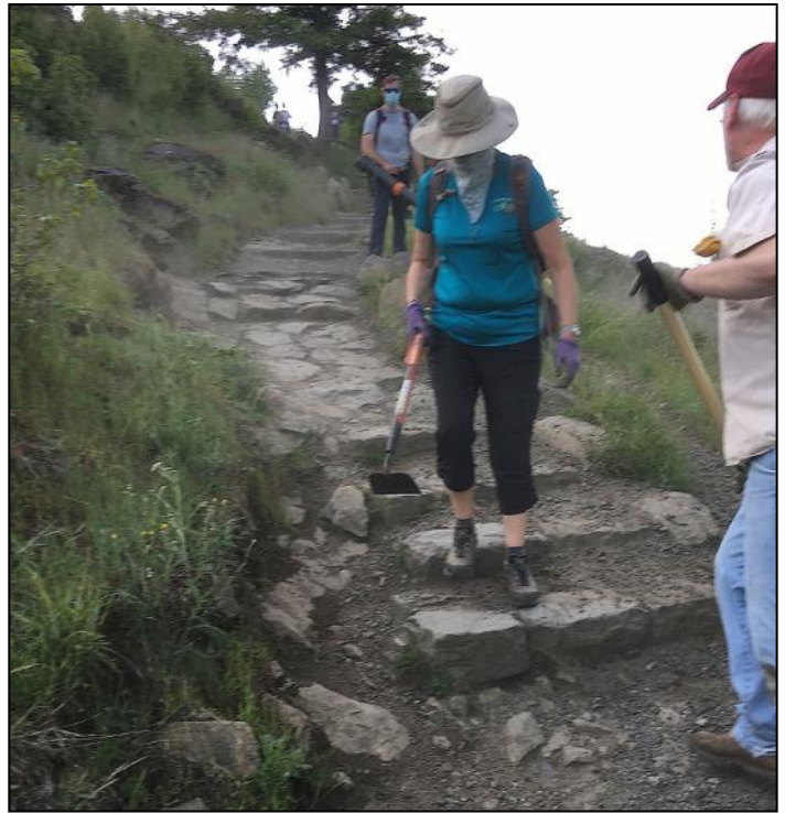
Jorry and Dan worked down from the top to dig out debris, gravel. Matt is behind with the blowers.
