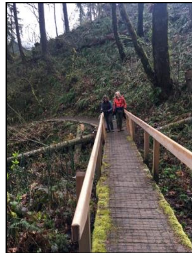
Damaged during the storm, the cedar handrails on the bridge below the Raptor Center have been repaired. Obsidians installed new handrails back in April and May 2022. Photo by Janet Jacobsen.
