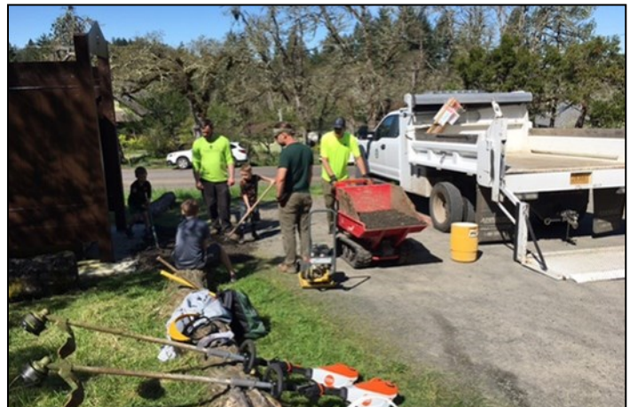
Janet's snacks, two trucks, motorized wheelbarrows, weed eaters, water, and more tools were needed to get this job completed.
