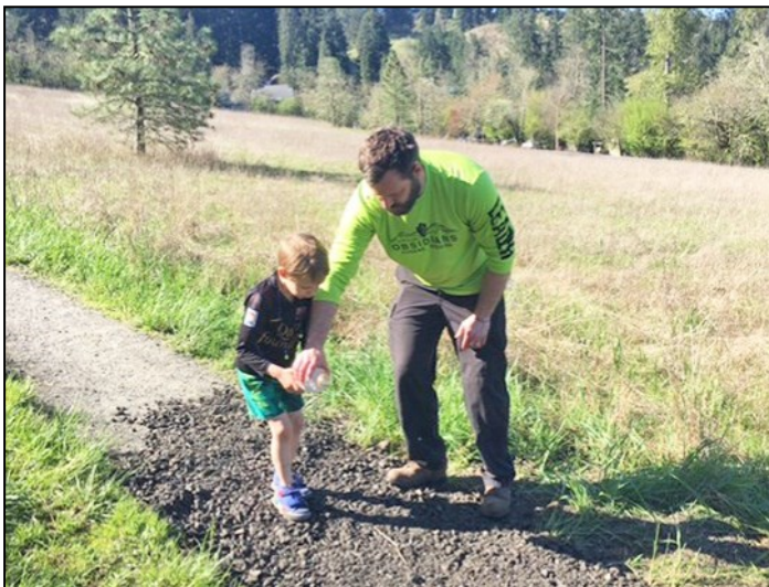
After the gravel is spread, Matt shows Fletcher how to spread water before they use the compactor.
