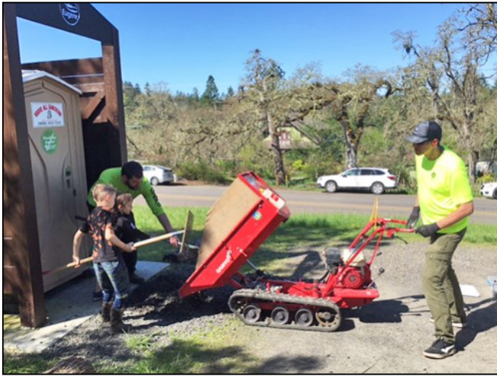
Josh dumps a load of gravel in front of the portable toilet. Matt, Nathaniel, and Fletcher prepare to rake.
