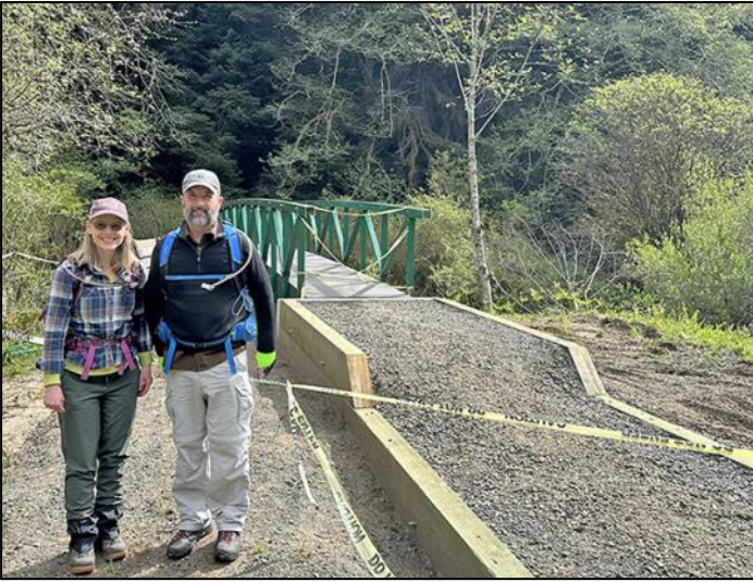
Kim and Bill by the nearly completed new bridge across China Creek. It won't be long before we can hike the Valley Trail again.
